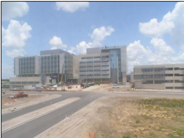
Figure 2 – Nemours Children's Hospital as a part of The Nemours Foundation. Courtesy The Nemours Foundation.
